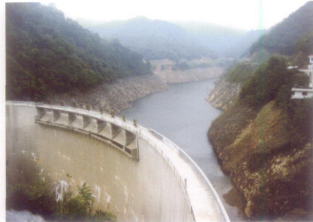
附图24 阳明山二级电站水库大坝及库内落水带水土流失情况
